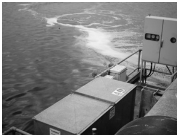
Figure 7: Oxygen injection into Salford Quays.
