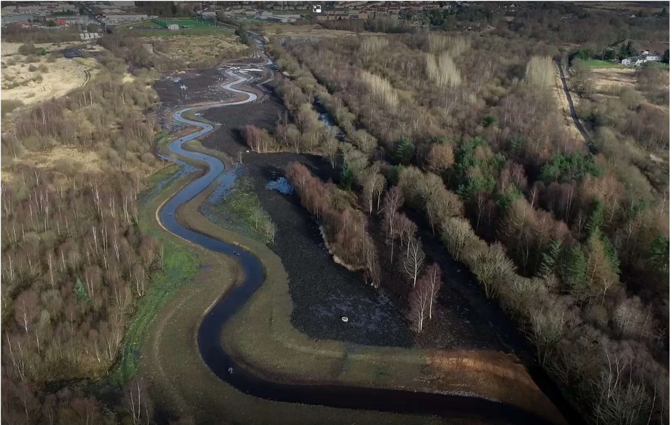
Drone footage of the Garrel Burn in March 2022, immediately after construction was complete.
