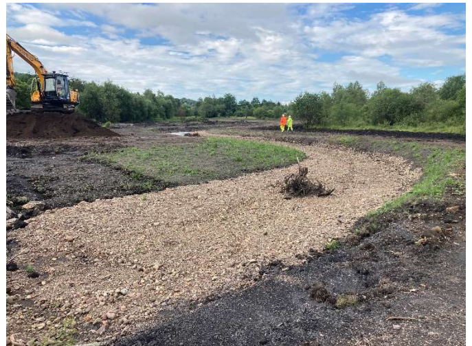
Lower reach of restored channel showing bar apex large wood structure during construction.
